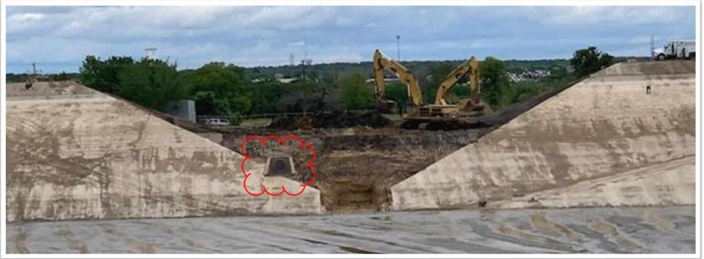
Actual location of 48" inlet piping, within excavation zone for new 10-foot diameter outlet pipe
