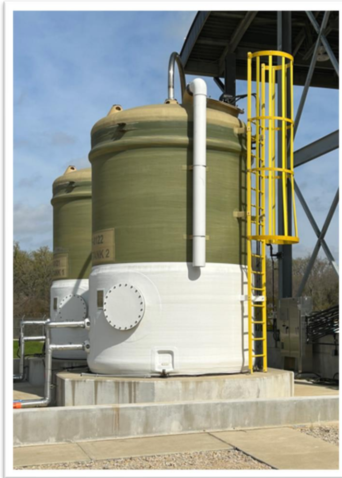
Salt storage tanks
