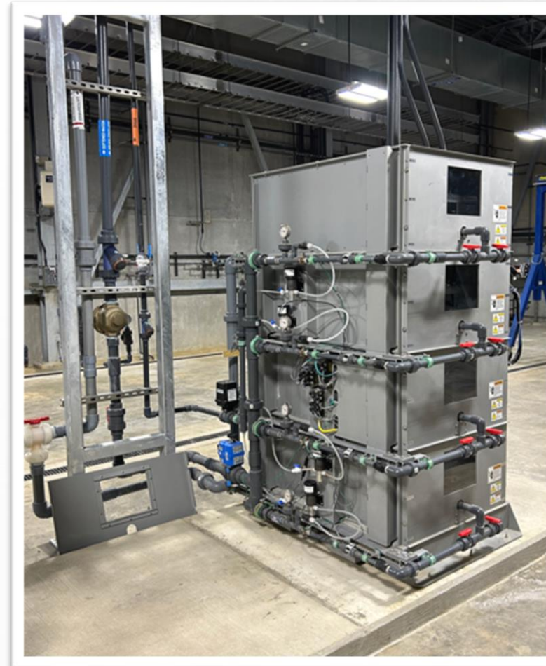
Salt (brine solution) used to generate sodium hypochlorite (bleach)
