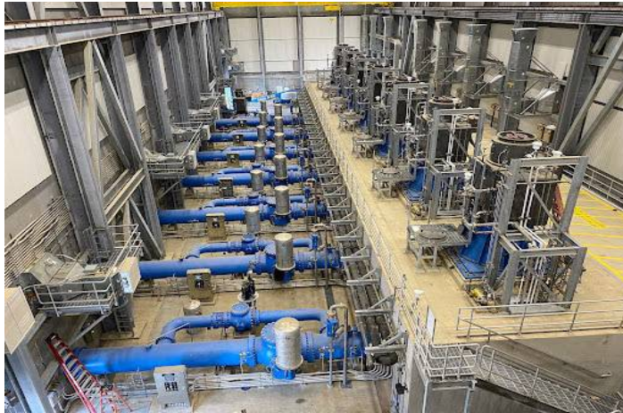
(JCC1 Pump Station at Cedar Creek Lake)
