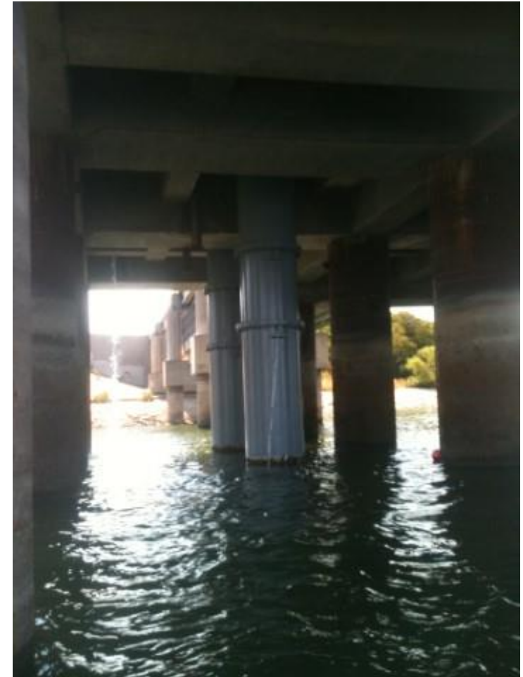
Pump Column Below
