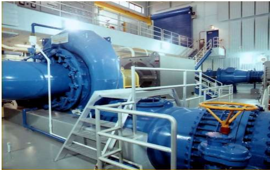
The Hydroelectric Turbine, pictured above, is located at Arlington Outlet and produces electricity which the District sells back to the grid.
