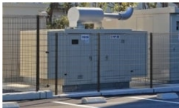
Emergency power generator
