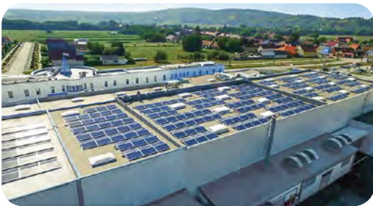
The photovoltaic system at our plant in Hungary.
