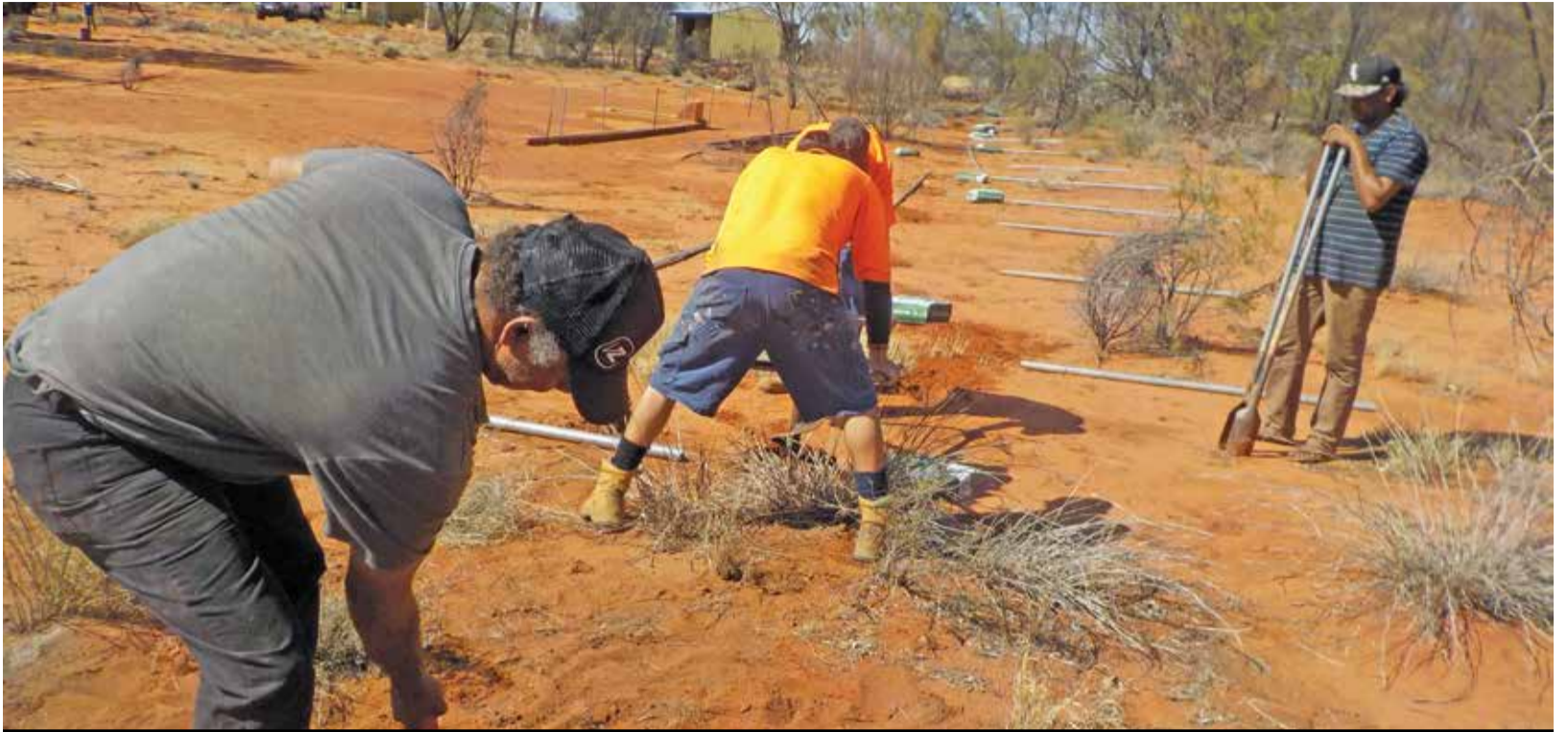
Graham Silverton (left) digs holes for fence posts at the West Waterhouse cemetery.
