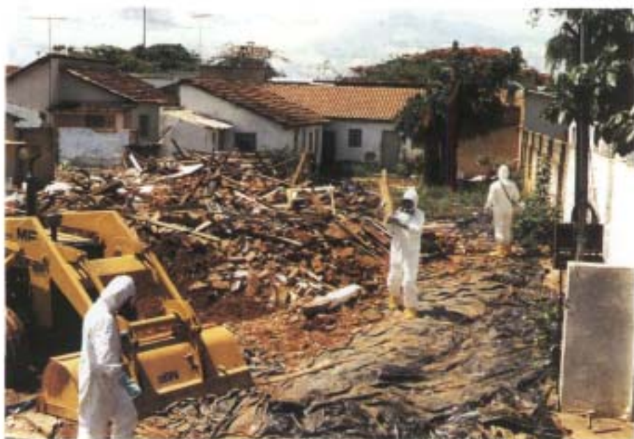
13. Contaminated rubble from the demolition of R.A.'s house on 57th Street.
