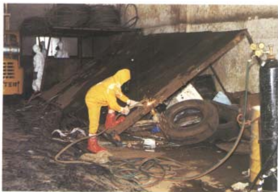
16. Cutting up contaminated items for removal from the warehouse of Junkyard III.
