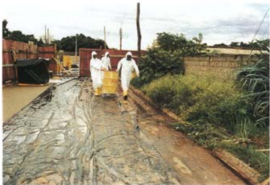
21. Much of the decontamination work had to be done in heavy rain.
