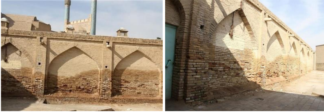
Figure 27. Increase in the humidity levels before the reorganization of the sewage networks
