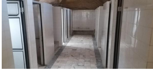
Figure 29. The previous condition of bathrooms in Masjed Emam with leakage issues and inauthentic design
